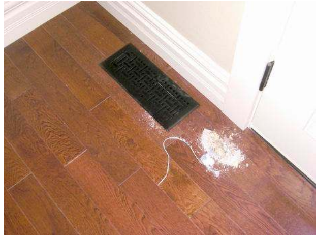
17 debris from register boot
