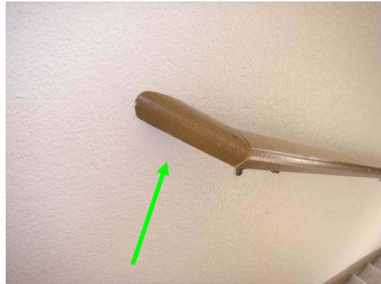
14 15 typical handrail with proper "return"
