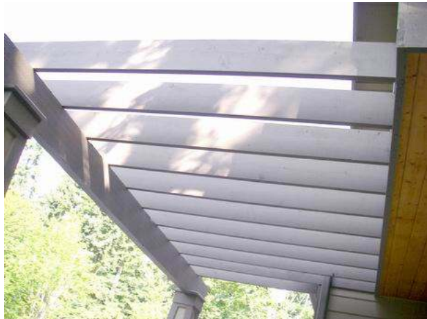
untreated rafters on pressure-treated beam
