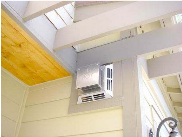
16 fireplace flue in close proximity to framing
