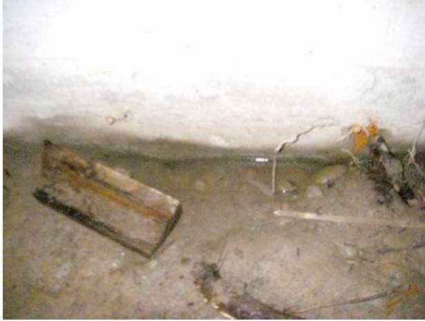
cellulose debris in crawl space
