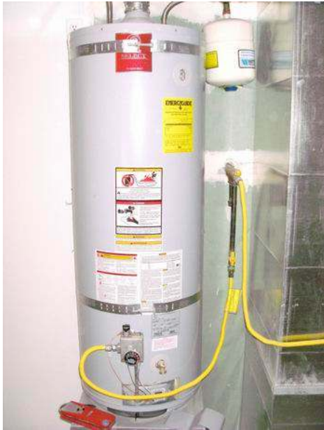
xx water heater
