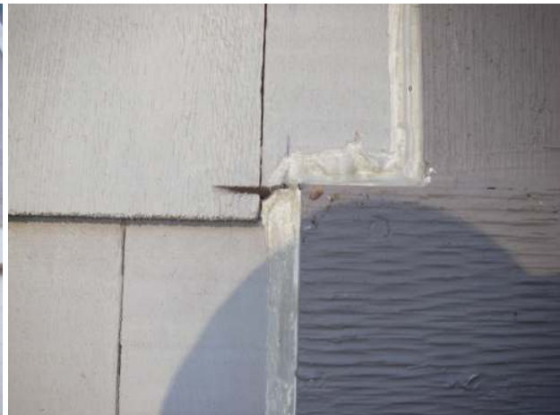
15 overcut and uncaulked shingle at window
