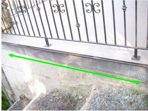
unfinished mesh on side of deck
