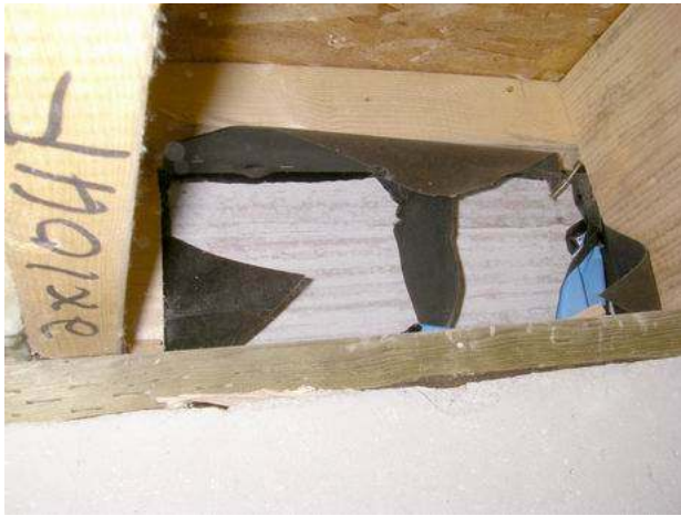
8 9 blocked crawl space vent
