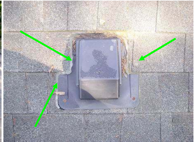
15 caulk at all fan duct discharge vents
