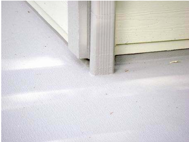
downspout penetrates deck membrane
