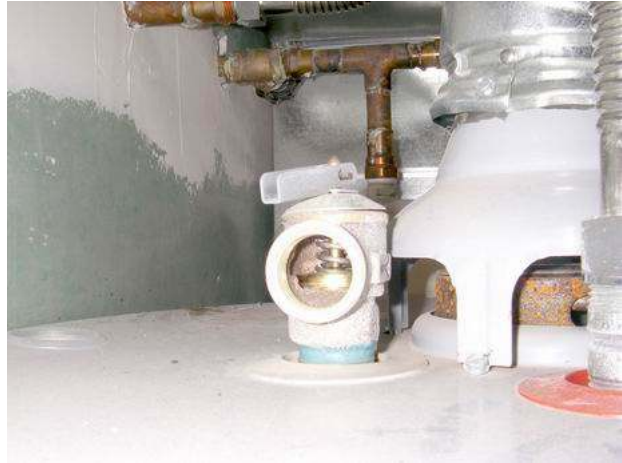
no discharge pipe from TPR valve
