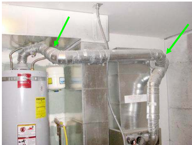
reverse slope (twice) in water heater flue
