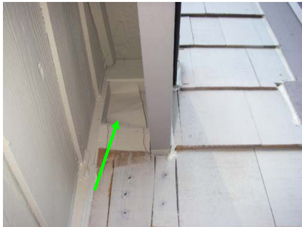
14 exposed building paper, not weathertight
