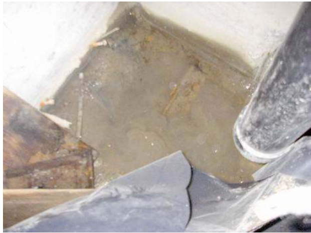
10 11 standing water in northwest corner
