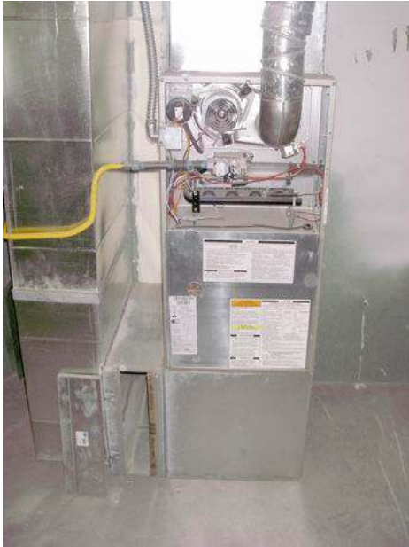
9 10 Payne/Carrier gas-fired furnace
