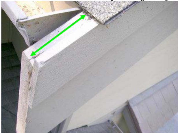
16 exposed barge rafter end
