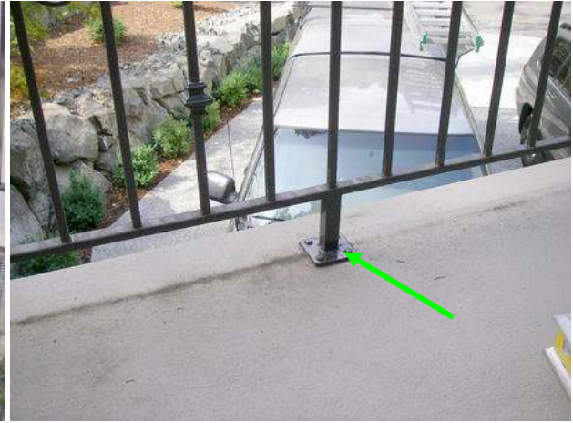
request confirmation that penetrations are sealed
