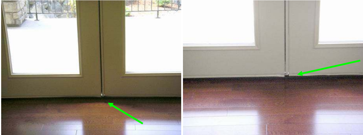
9 10 doors not weather-tight
