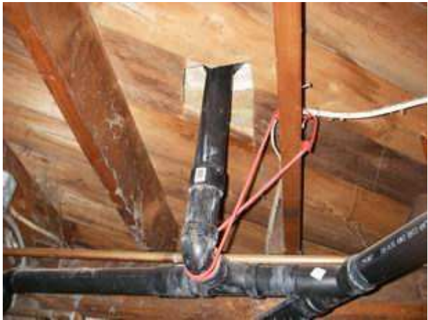
15 no P-trap at shower drain (note pipe hanger)
