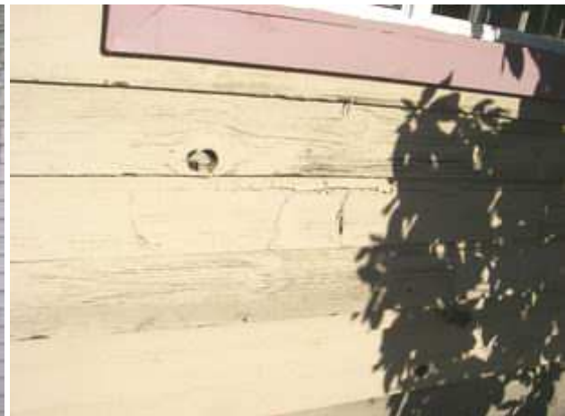
27 deteriorated clapboard siding
