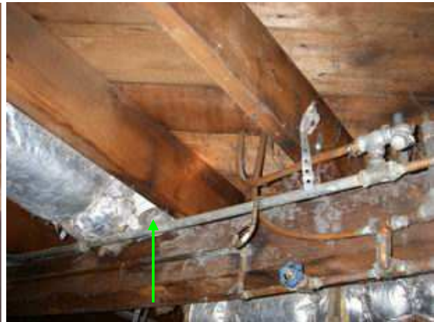
18 dryer duct discharge
