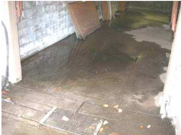
10 11 ponded water in basement (pump under grate)
