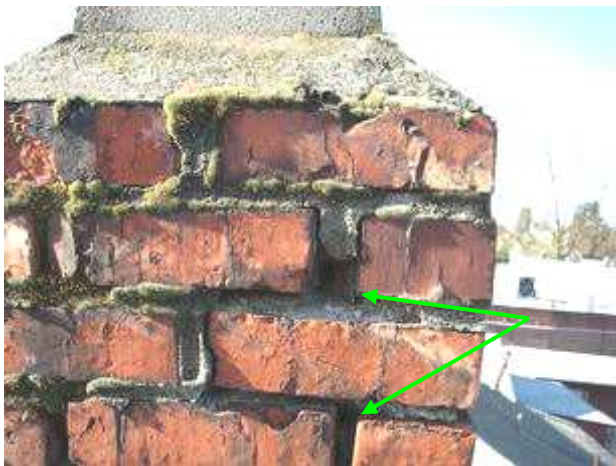
15 deteriorated mortar in chimney
