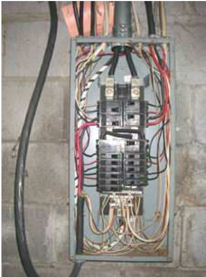
19 20 General Electric circuit breaker panel
