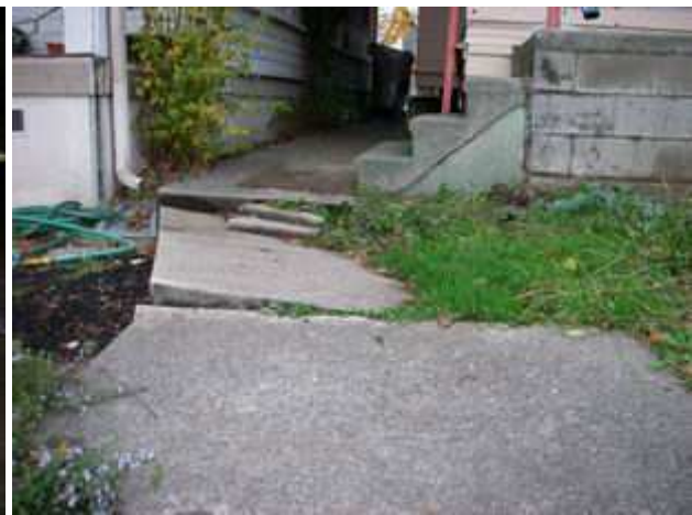
15 16 trip hazard near front porch
