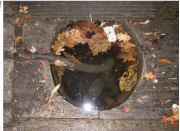
non-functional sump pump
