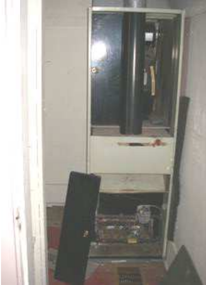
Payne naturally-aspirated furnace in bedroom closet
