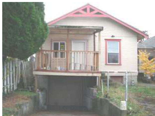
sagging, swayback and un-level deck
