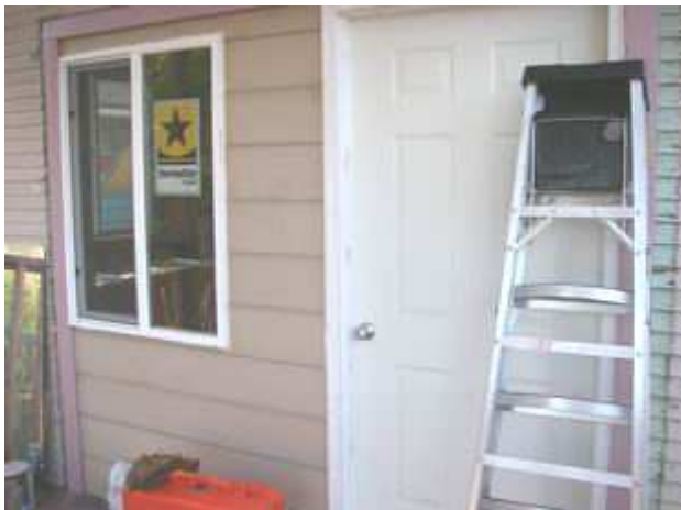
26 T-1-11 siding mounted sideways
