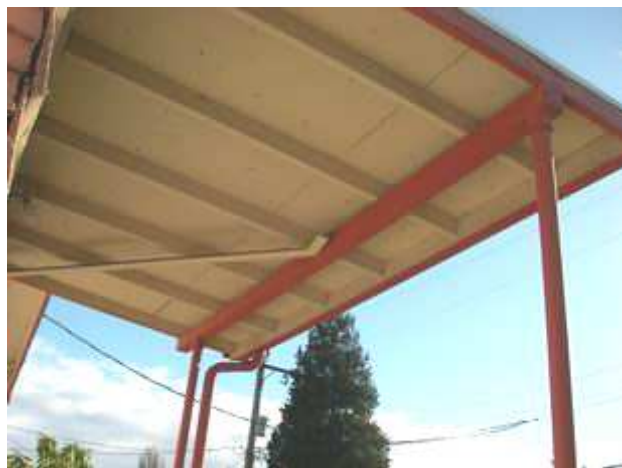
substandard porch roof framing
