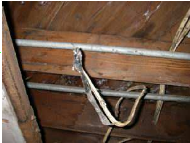
13 “live” conductor not properly terminated
