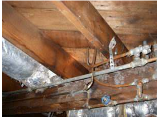
copper and galvanized water supply lines
