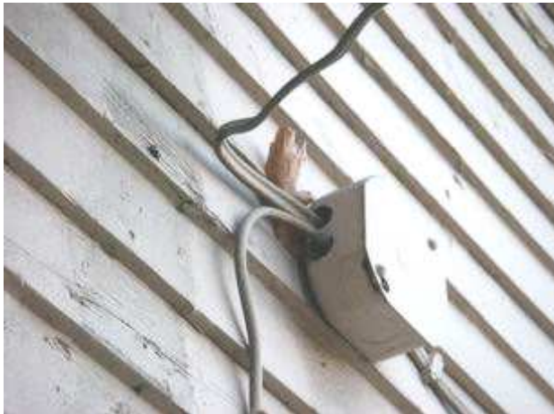
14 improper wiring (materials and methods)
