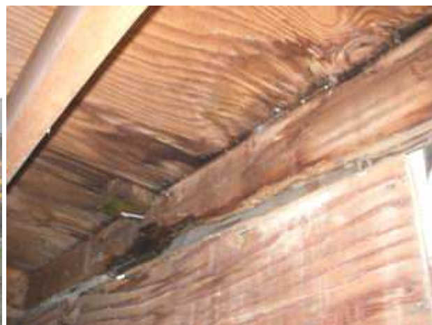
decay in deck framing
