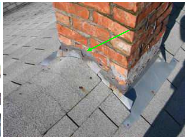
16 moisture intrusion at missing counter flashing
