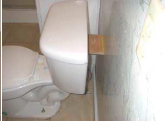
11 wood block supporting toilet tank
