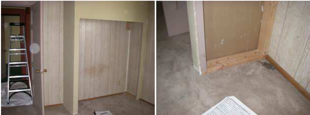
10 11 unfinished closet with substandard framing built on top of carpet with 5' 10" high opening 12 13
