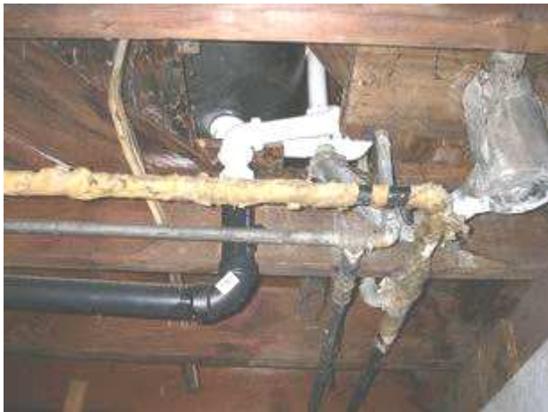
14 convoluted waste piping with no P-trap
