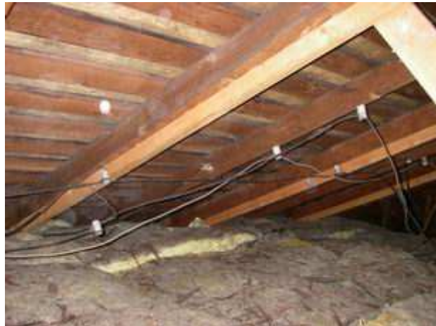
21 22 “live” knob and tube wiring in attic
