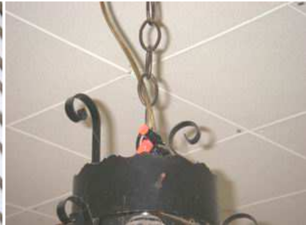
15 improper interior lamp splicing
