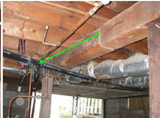
26 excessive beam cantilever
