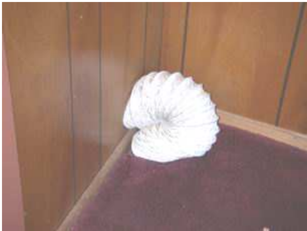
17 dryer duct routed through bedroom
