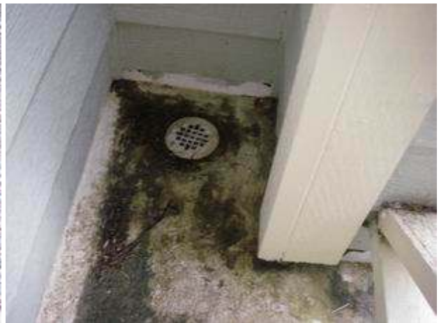
drain grate over entry (see below)
