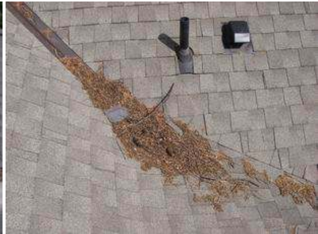
organic and construction debris
