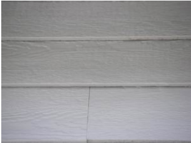
butt joint uneven & not caulked
