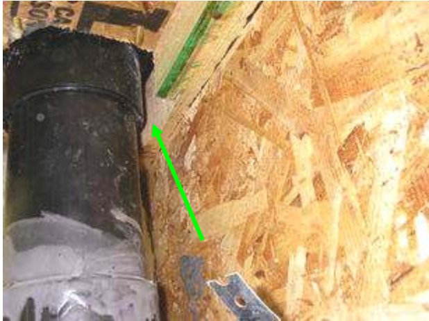
notched top chord
