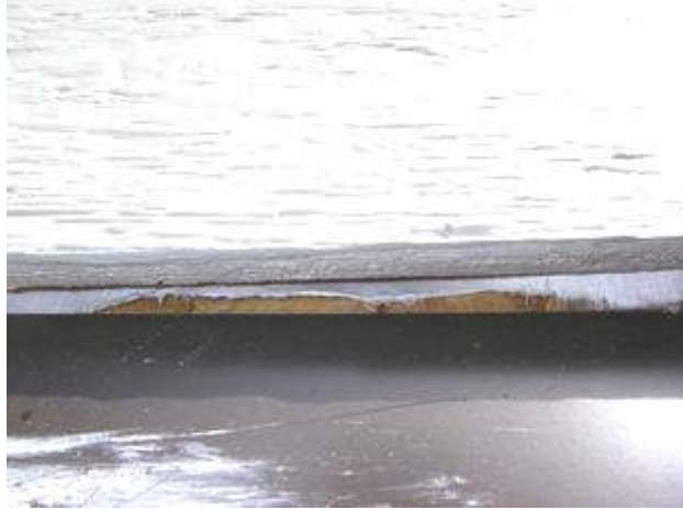
exposed sheathing above roof-to-wall flashing
