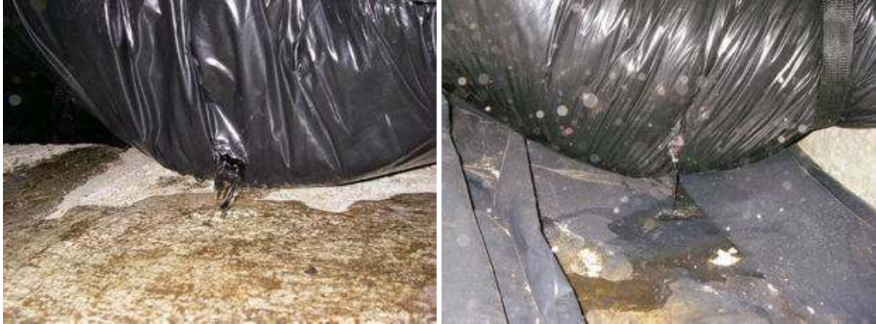
2 3 heat ducts blocked by accumulated water
