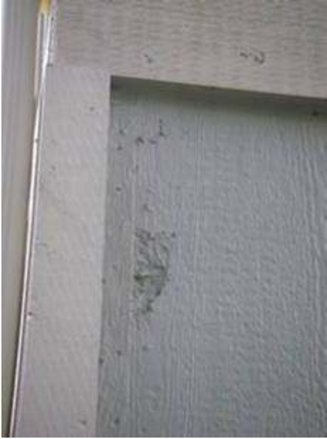
damaged siding skin
