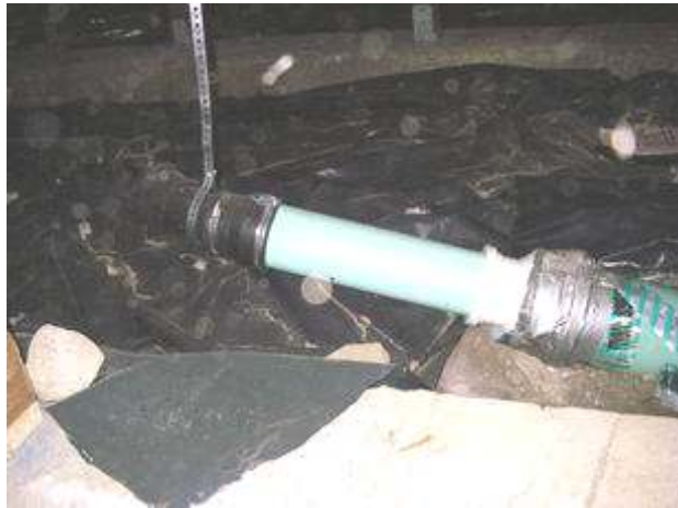
6 7 “spliced” sewer pipe
